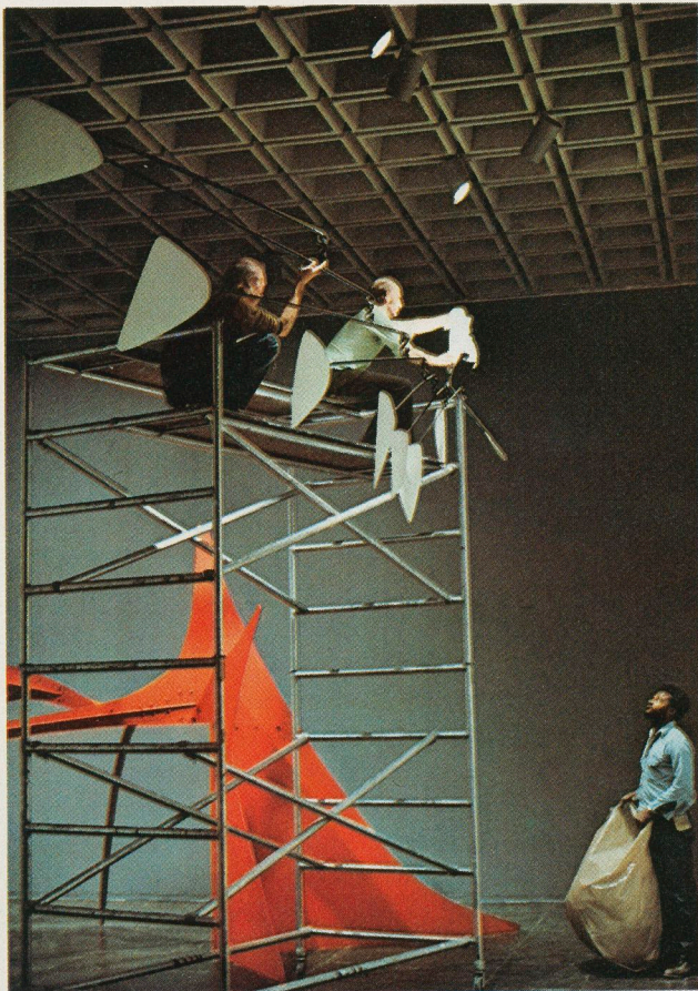
Museum technicians work on elaborate scaffolding to install Calder mobile to its best advantage.
